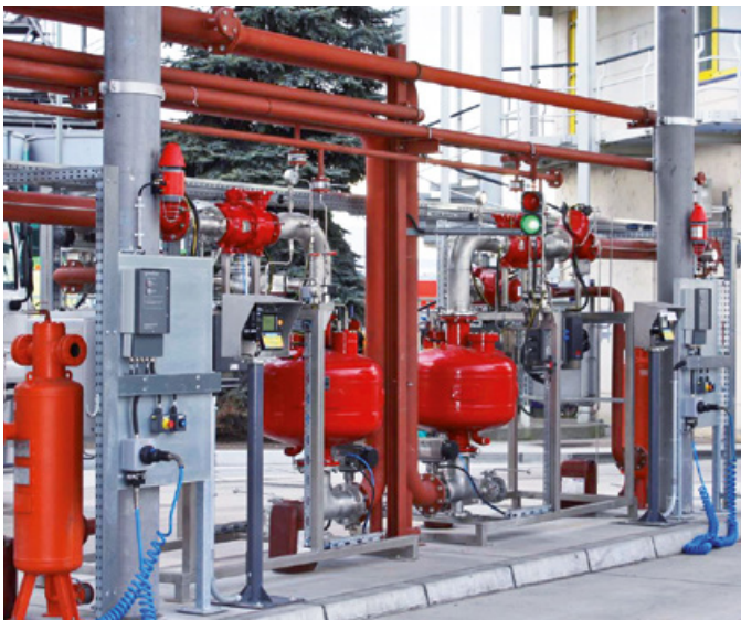
↑ CMS: compact metering skid
